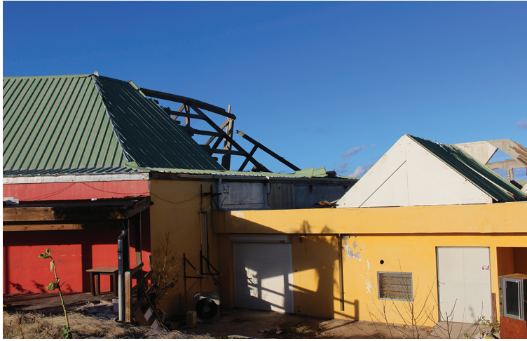
Figure 5: Incorrectly braced frame
