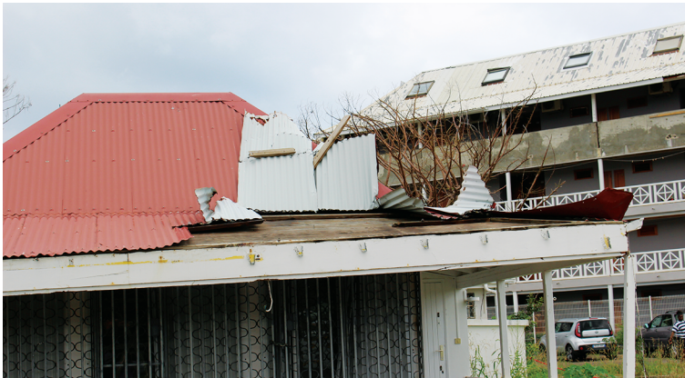
Figure 6: Uplift of the roof edge – sheet too thin and insufficiently steep, insufficient fastening causing perforation
