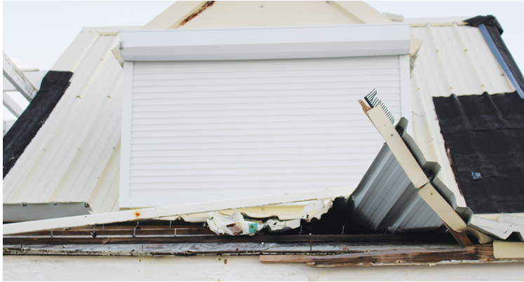
Figure 3: Batten with cross section that is too small and/or is fastened insufficiently
