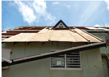
Figure 3: Purlin spacing too wide
