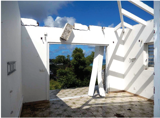
Figure 13: Improper assembly of the masonry and lack of bracing on a hip roof frame
