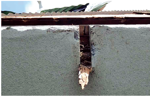
Figure 10: Bad frame-to-wall tie fixing
