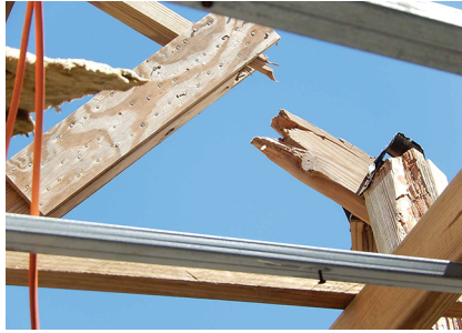
Figure 2: Cross-section not substantial enough
