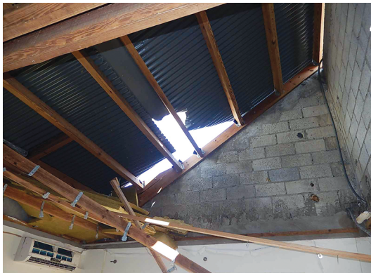
Figure 6: Bad panel-to-purlin fixing
