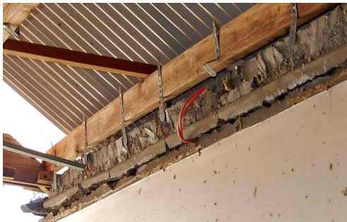
Figure 11: Improper attachment (flats poorly anchored)
