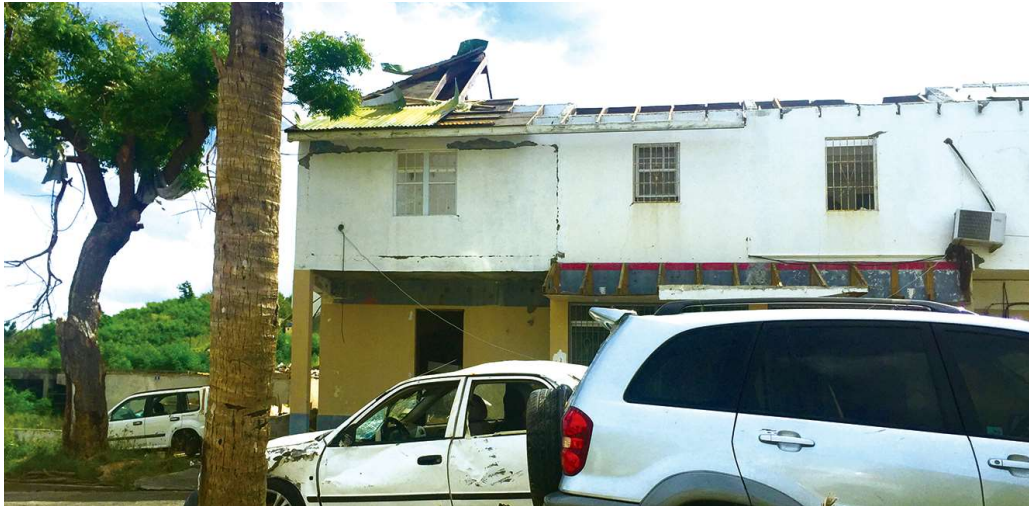
Figure 2: Damaged structure at the confining elements
