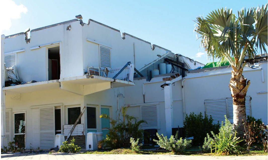
Figure 3: Breaks due to the frame being ripped out
