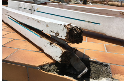
Figure 6: Posts with ripped out right-angled fixing brackets
