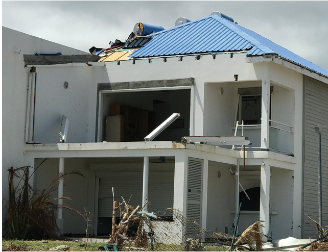
Figure 1: Awning ripped off
