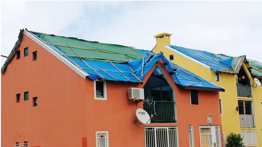
Figure 1: Damage to roofs
