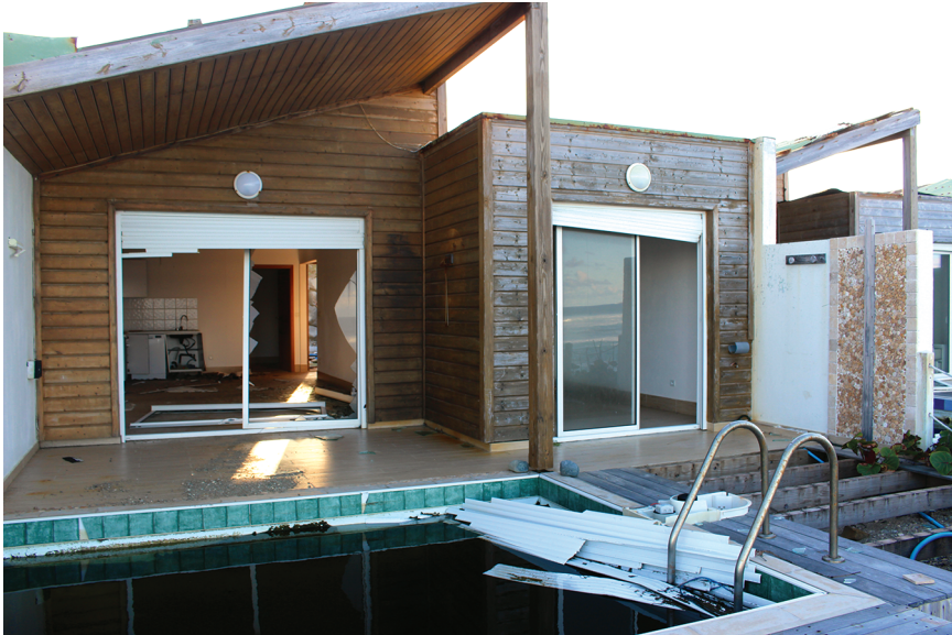
Figure 2: Damage to patio doors
