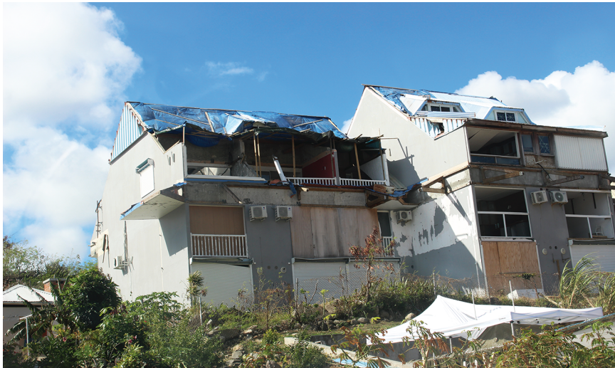
Figure 3: Damage to lighter sections of masonry buildings
